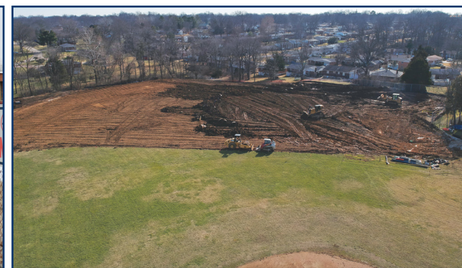
Work continues on the Mehlville High School ballfield. The previous field had grading issues and stormwater covers in the outfield.
