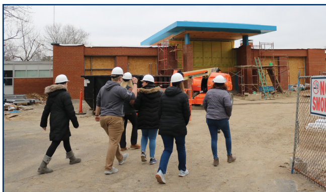
Construction is on schedule at Bierbaum Elementary School. The new entrance should be complete this summer.
