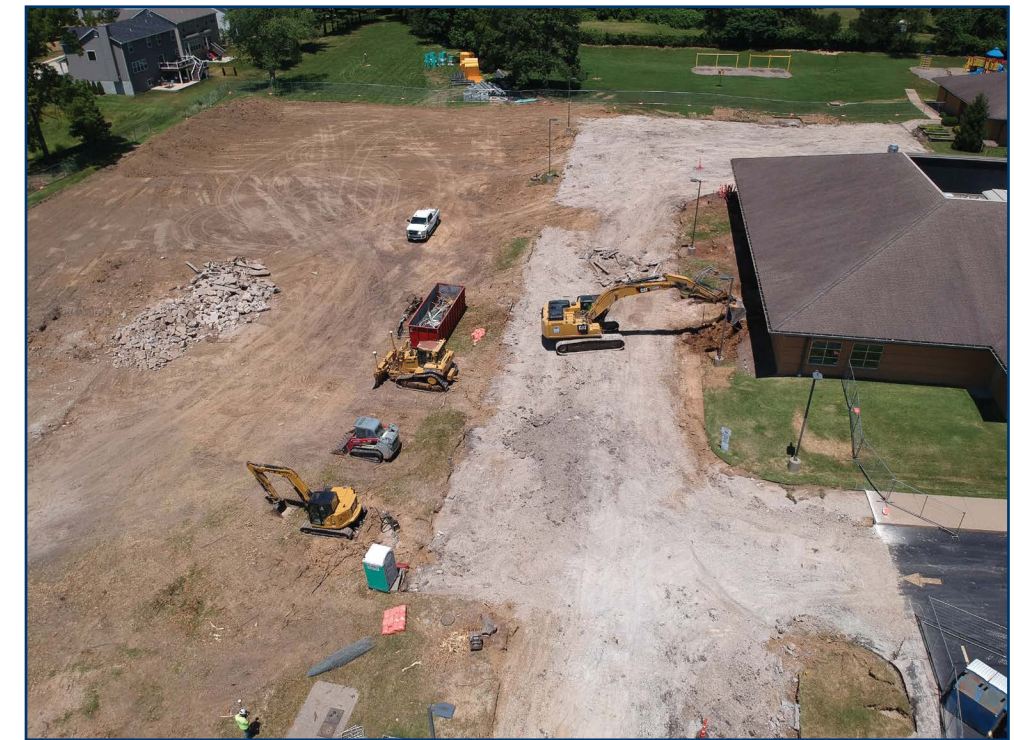
The Oakville Elementary parking lot is being expanded to improve student safety and reduce traffic congestion on Milburn and Yaeger roads.
