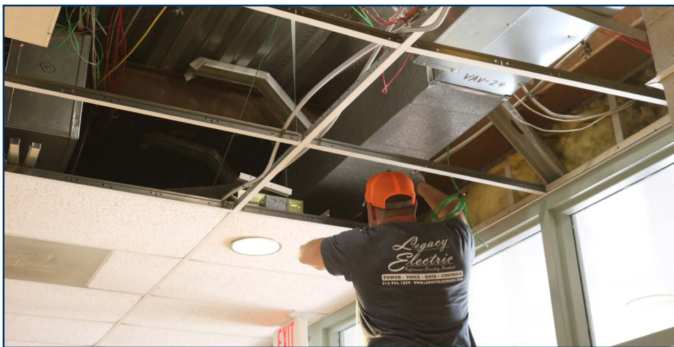
Crews finished a complete renovation of the heating, ventilation and cooling system at Forder Elementary School over the summer. The systems on the rooftop were replaced, as well as the boxes and thermostats in each of the classrooms and the diffusers in the ceilings.
