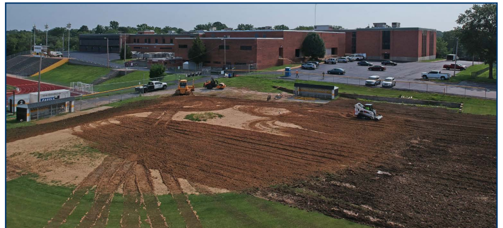
Crews are expected to complete extensive safety improvements to the Oakville High School baseball/softball field near the end of October.
