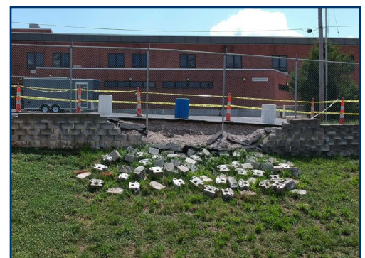
A portion of a retaining wall near the Oakville High School football stadium collapsed during the spring. Crews replaced and reinforced that wall over the summer.
