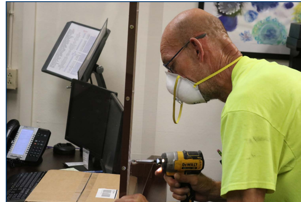
Carpenter Scott Lancaster installed plexiglass barriers in high traffic areas, like school offices and cafeterias, to help keep staff safe when students and visitors return to school.
