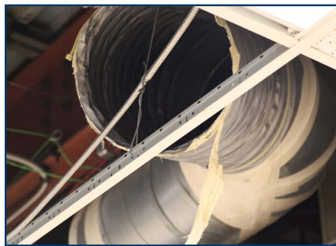
The HVAC system at Hagemann Elementary School was replaced this summer including new controls and wiring throughout the building.
