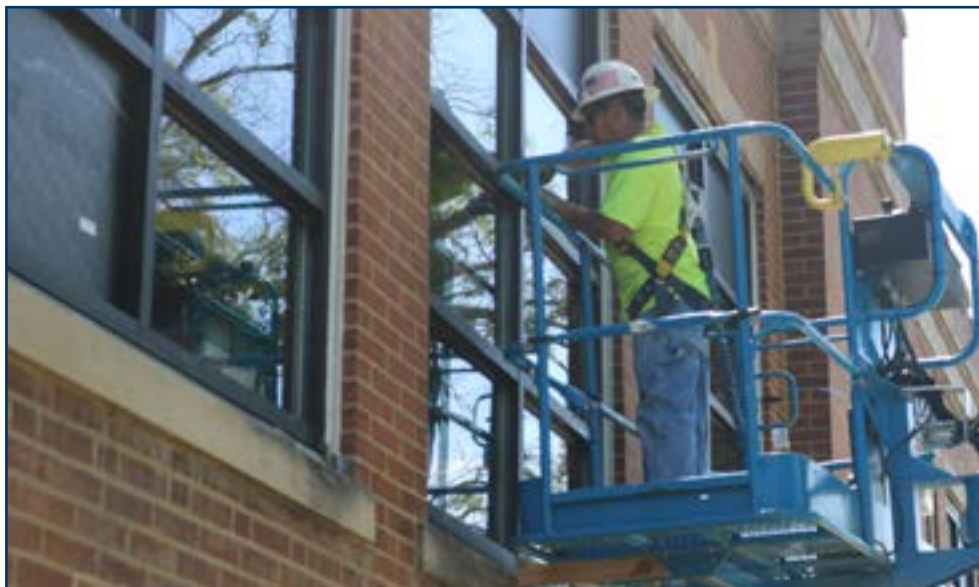
Workers install new energy-efficient windows at MOSAIC Elementary in July. The school also received new heating, ventilation and air conditioning.
