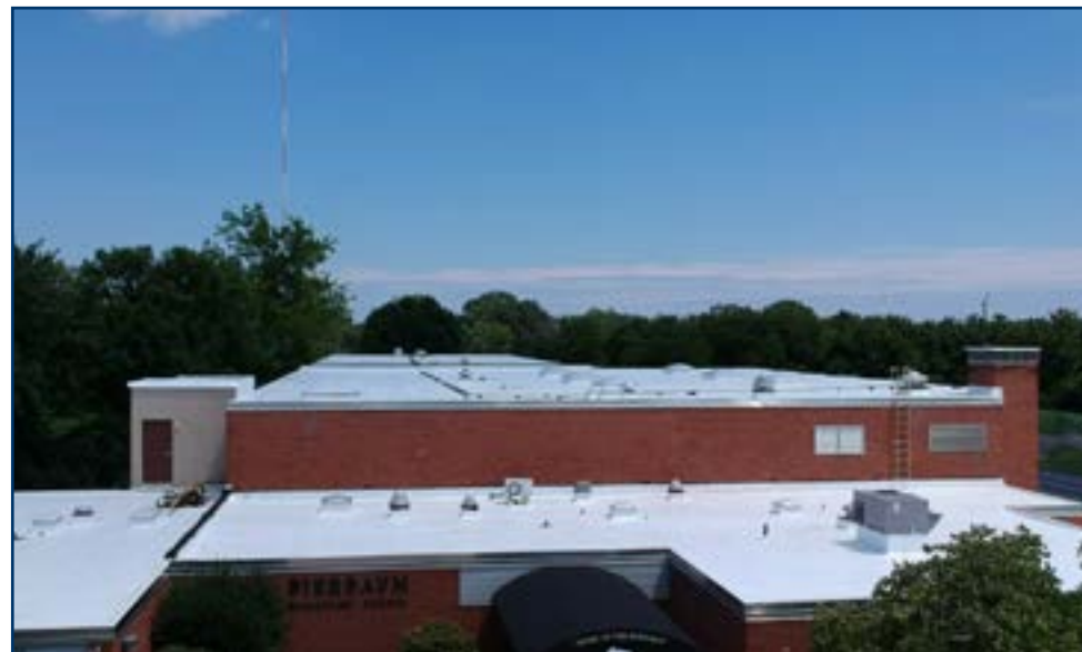
Bierbaum Elementary’s leaky roof was replaced this summer. Not only will this new roof make school more comfortable for students and staff, it is also more energy efficient.
